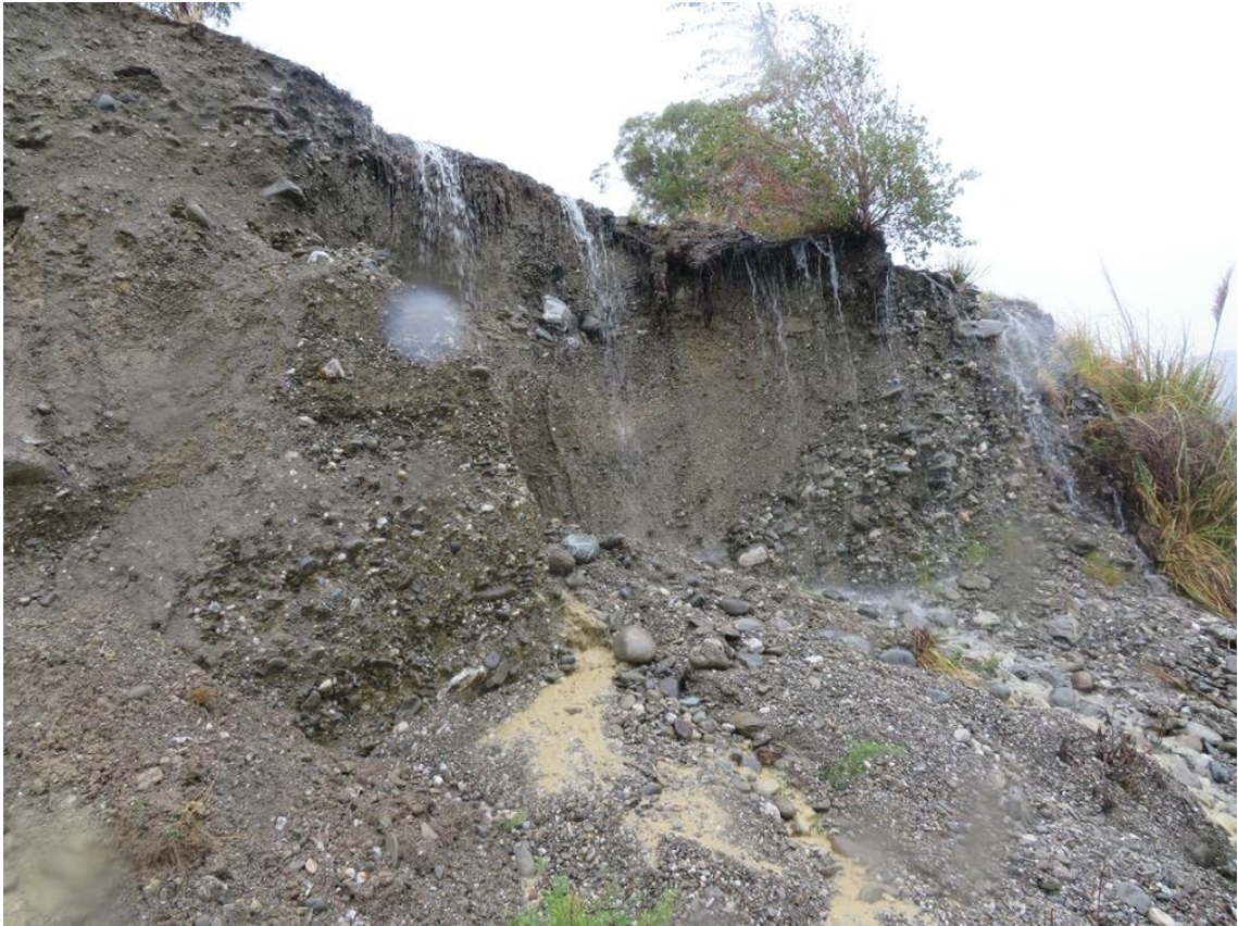
Fig 5. Flora Dora Cliffs directly north from stormwater drain
