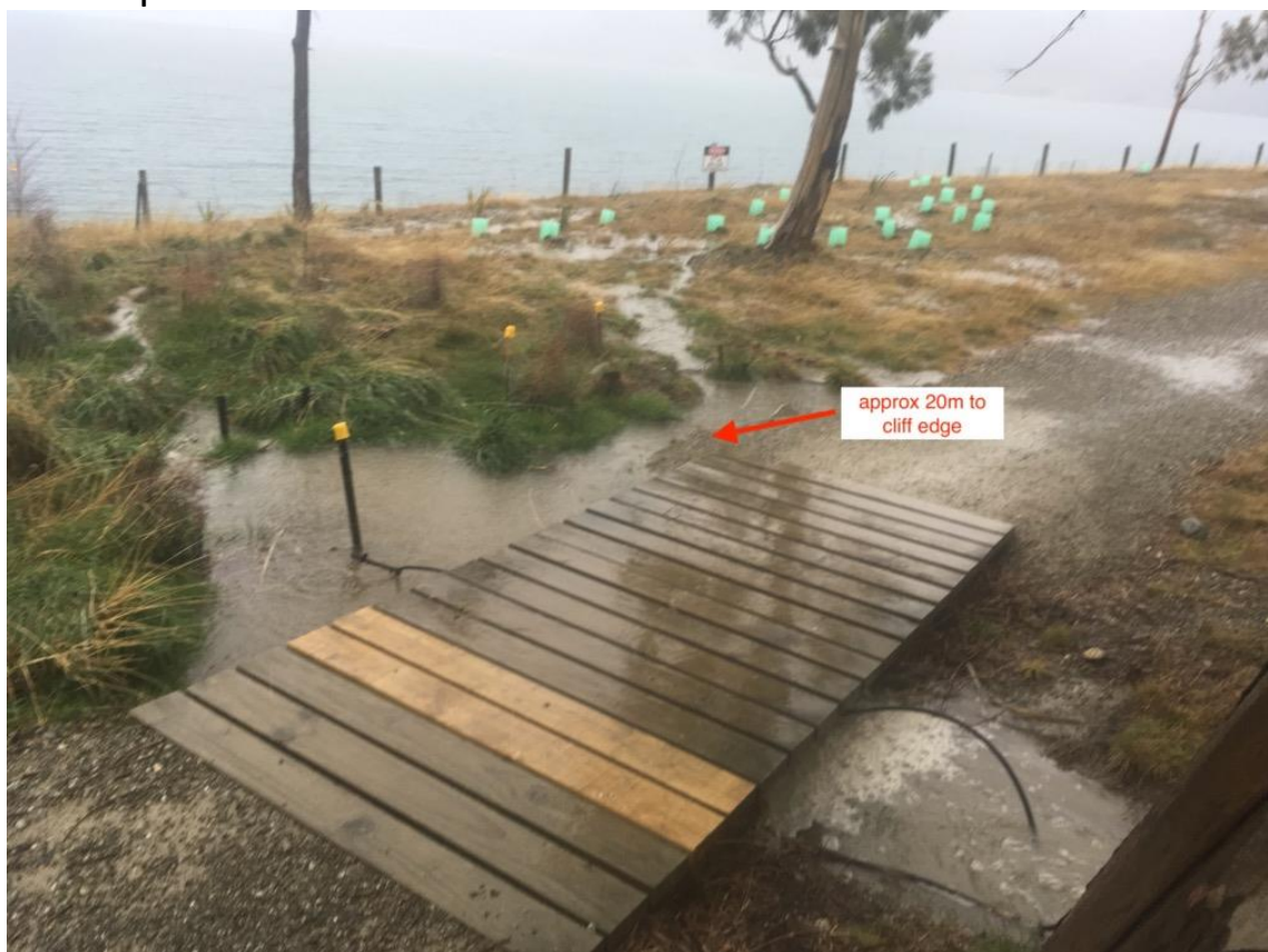
Figure 4. flooding on Flora Dora terrace arising from open storm water drain. The boardwalk is on the Gladstone track
